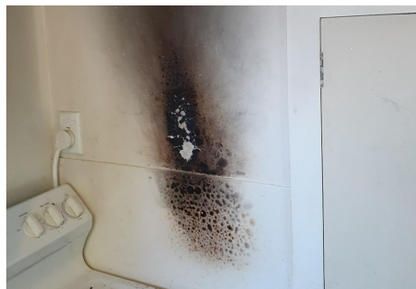
Small stove fires can cause unseen damage
